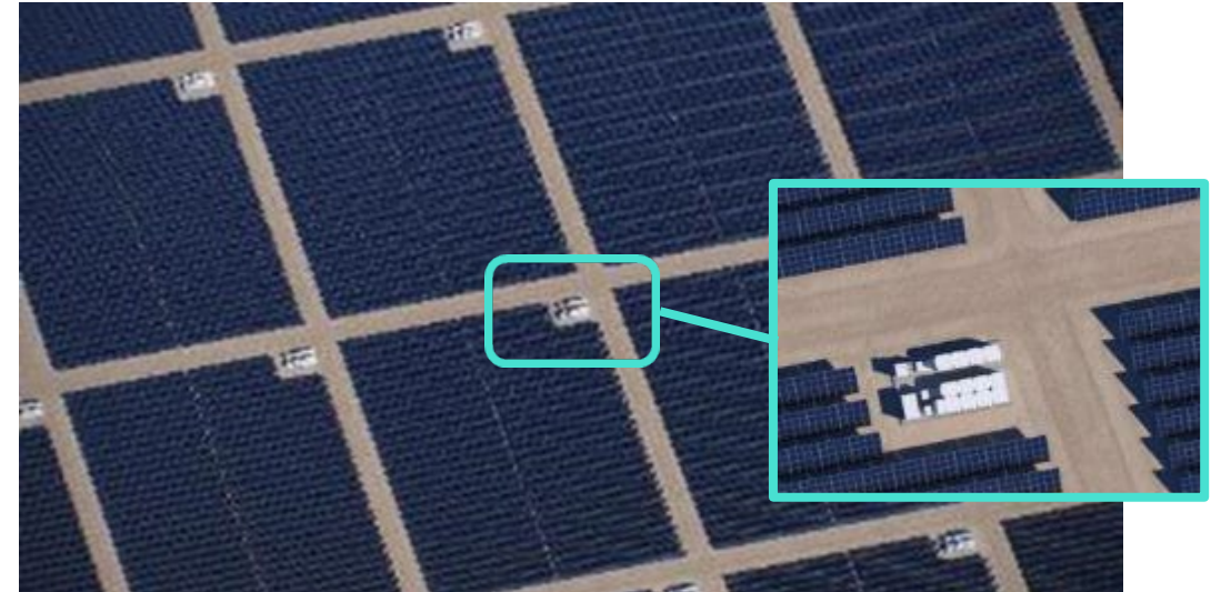
Storage system distributed within PV field
