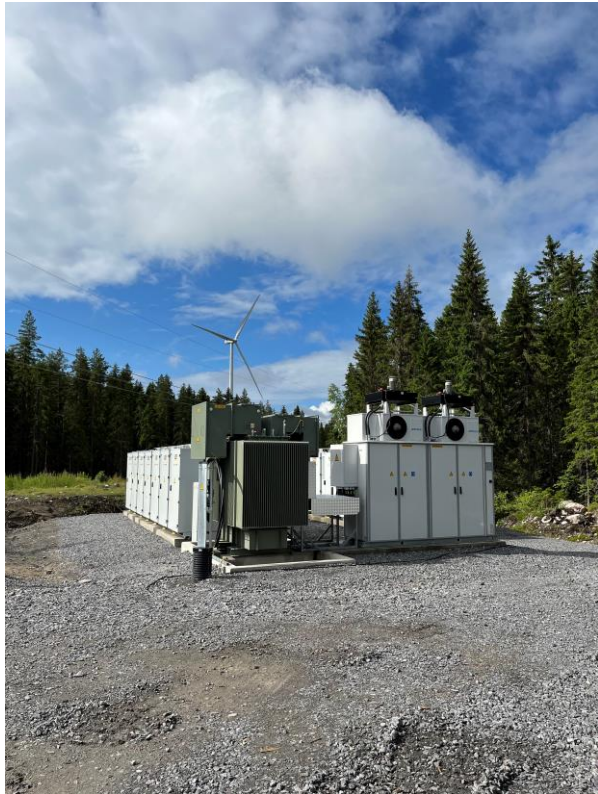
July 2023 Hot commissioning
